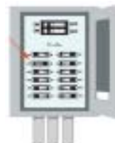
Circuit Breaker Box
